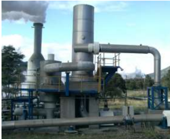
TOPP1 Geothermal Steam Separator
