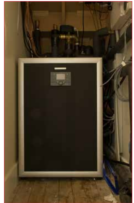
Quiet and unobtrusive, the heat pump unit is stored underneath the stairs.
