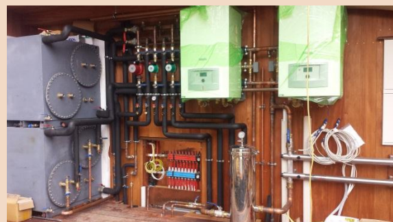
Bosch equipment graces the plant room
