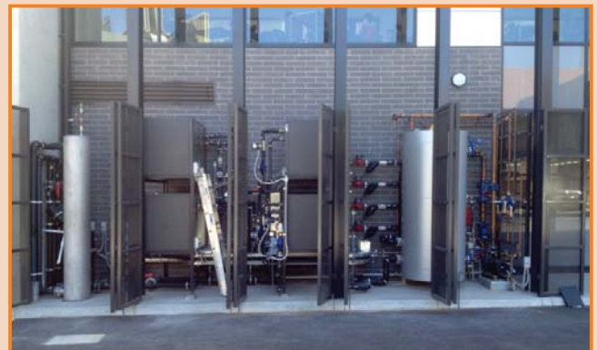
Enclosure for heat pumps, control & distribution system & buffer tanks
