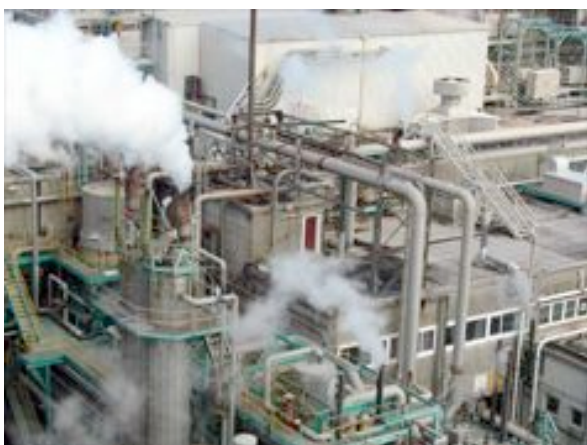
Figure 5: Geothermal supply main and stripper towers (Photo courtesy of CHHT from www.teara.govt.nz ).
