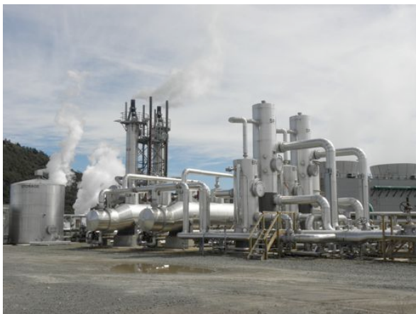
Figure 7: NTGAL's SCA supply clean steam plant
