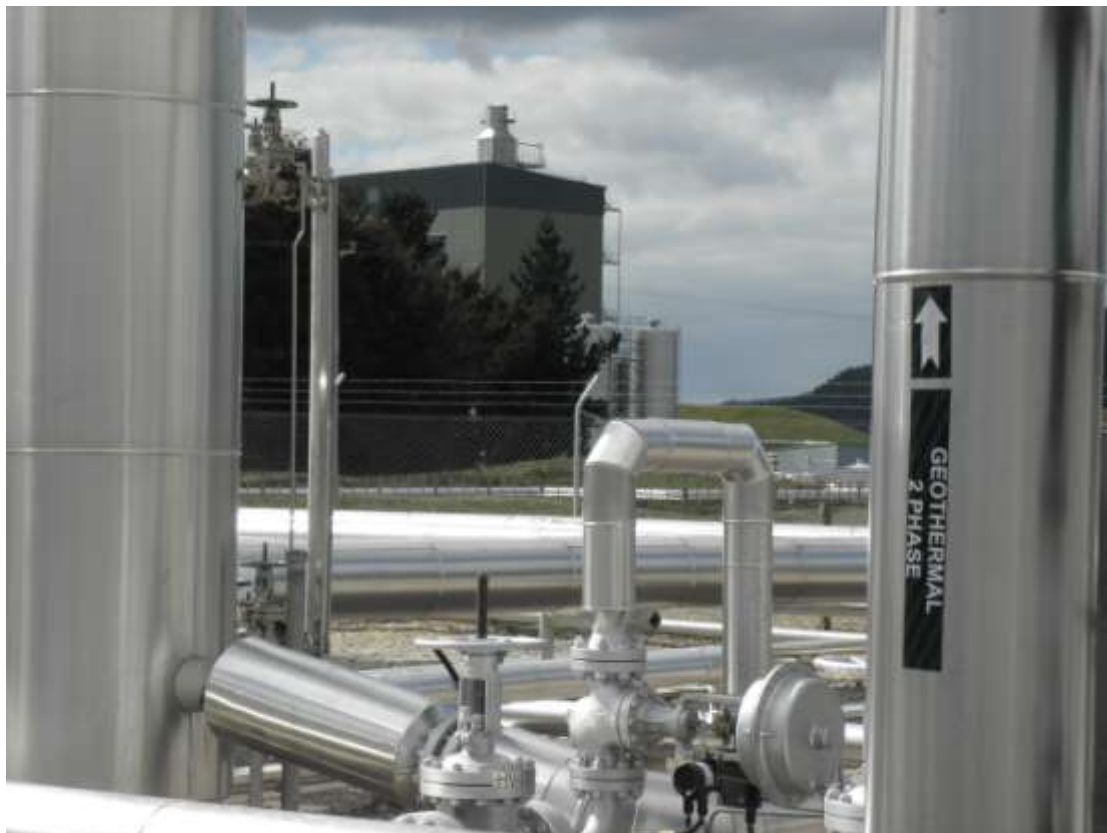
Photo: View from heat supply system through to the Miraka factory (from Andy Bloomer).
