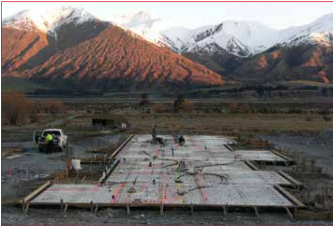
The under floor heating circuits.
